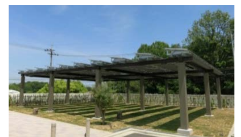
Solar power equipment (17.1 kW) over regulating reservoir (common area)
