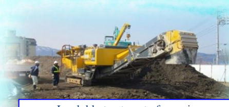
Insoluble treatment of arsenic-contaminated soil Private hospital Insoluble treatment of arsenic-contaminated soil on the premises of a hospital
