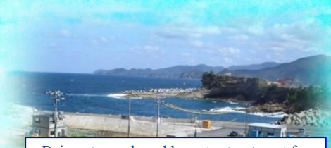
Rainwater and muddy water treatment for site-preparation work Chugoku Electric Power Construction of the Shimane Nuclear Power Plant Unit 3
